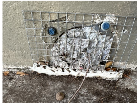
Screen plugged w/debris
