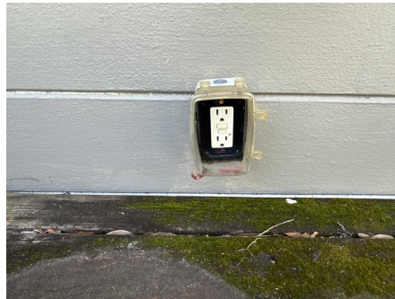
Also missing cover
