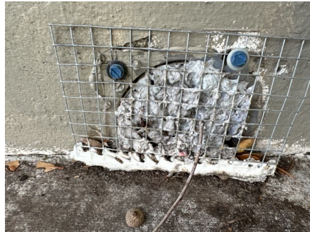
Screen plugged w/debris
