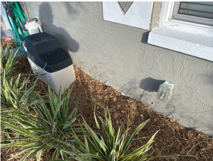
Extension cord used for water softener
