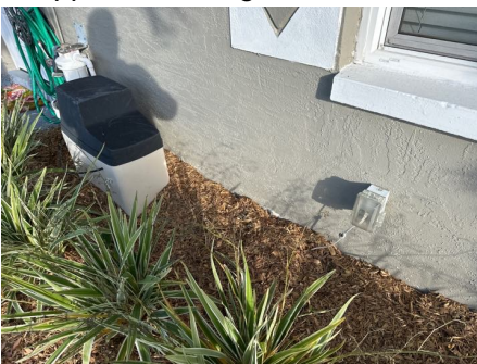
Extension cord used for water softener
