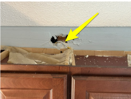
Above microwave cabinets
