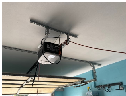
Extension cord used for garage opener
